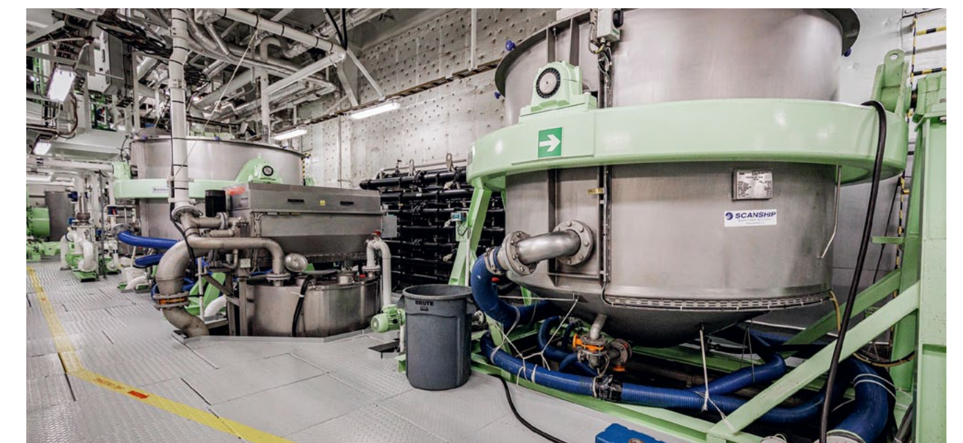
Wastewater treatment on board
